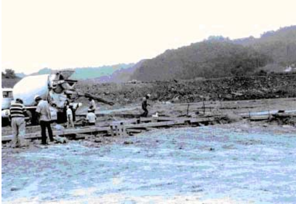
Figure 6. Pouring footings at the Red Onion site after site stabilization. The surcharge fill is visible in the background of the photo.
